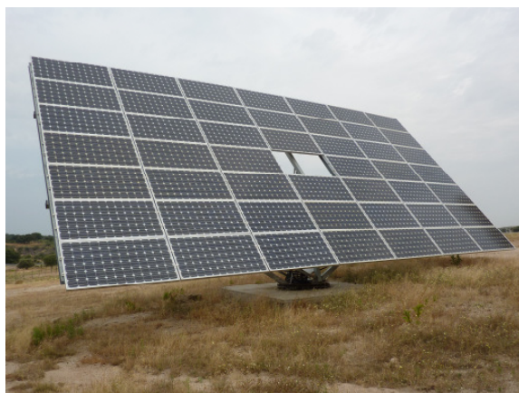
PV-Anlage in Albuquerque
