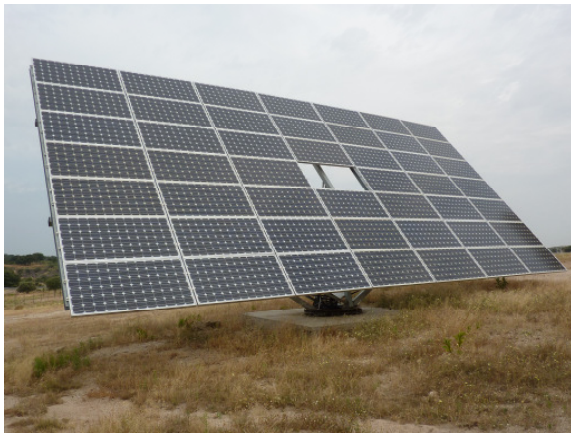
PV-Anlage in Albuquerque
